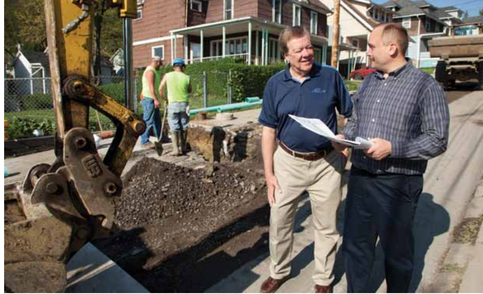
Dennis Stidinger, President of The EADS Group, and Project Engineer Steve Sewalk review a sewer lateral replacement project in Johnstown’s Roxbury neighborhood.
